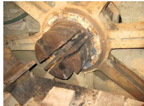
Shaft end showing wear
