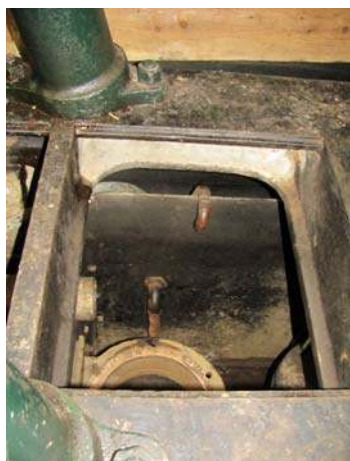
Small engines' condensate system pipes
