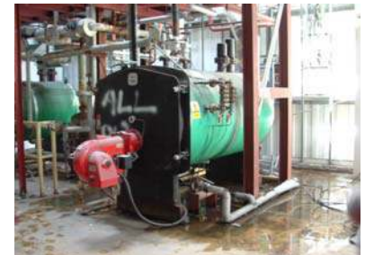
Wellman Robey Sygnette boiler located in the Sony factory at Bridgend
