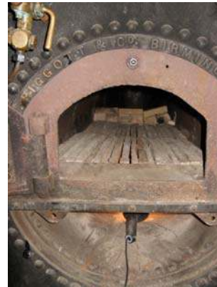
Cornish boiler front
