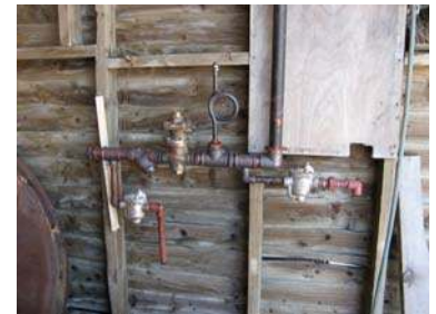
Steam main with PRV near new boiler
