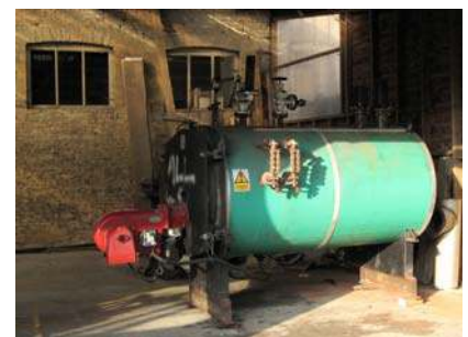
Sygnette boiler located in the lean-to at Combe
