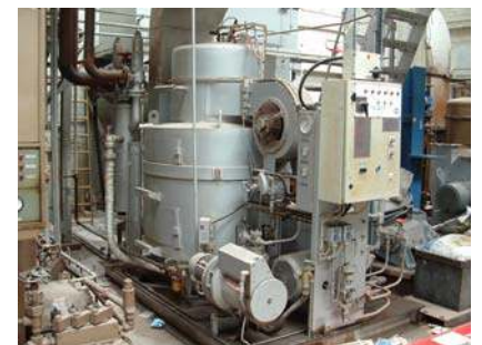
Stone Vapor flash steam boiler at Liverpool University May 2005
