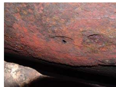
View of the drilled hole from flue showing minimal thickness of iron November 2004
