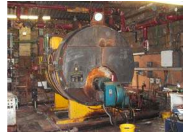
The B&E boiler at the mushroom farm Note the Coke can be on the burner indicating size
